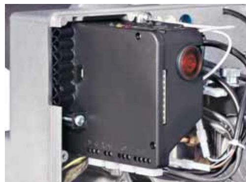
Control box fitted with ignition transformer
